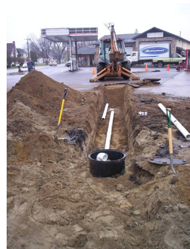
Free Product Recovery Installation
